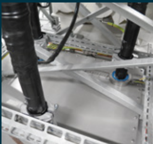
5. High voltage cables
