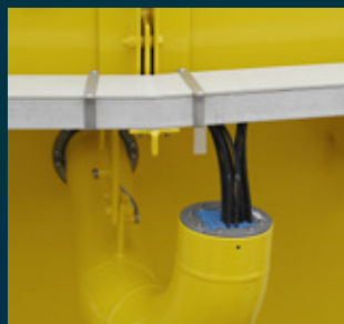
3. Deck equipment cables
